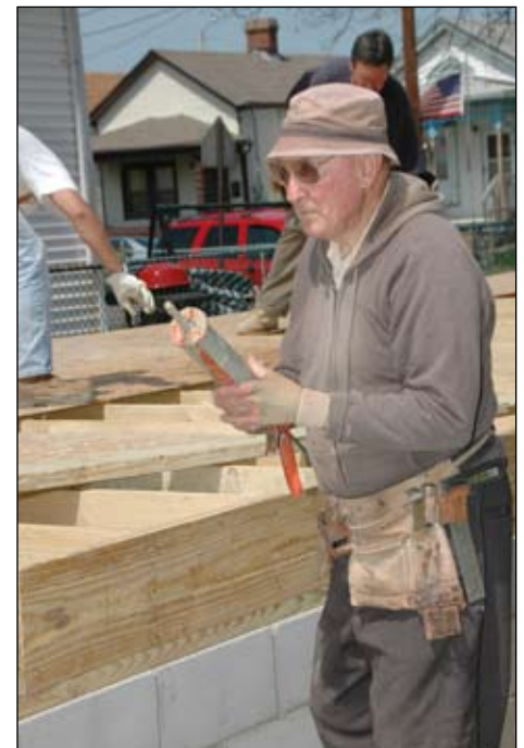
305 Houses and counting Volunteer Norb Carey, a volunteer since 1986, serves as a framing crew chief. "My job is to keep everybody busy." (Photo by Bill Sheets)
